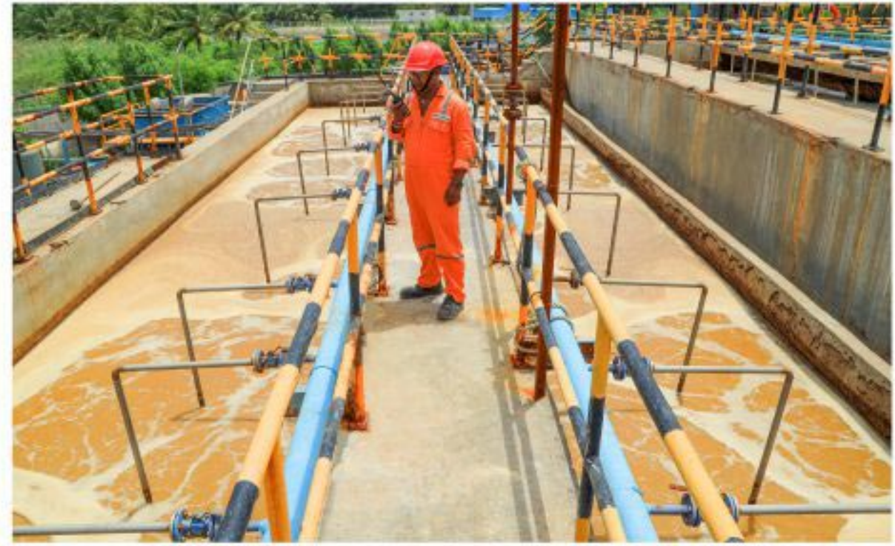
Effluent Treatment Plant
